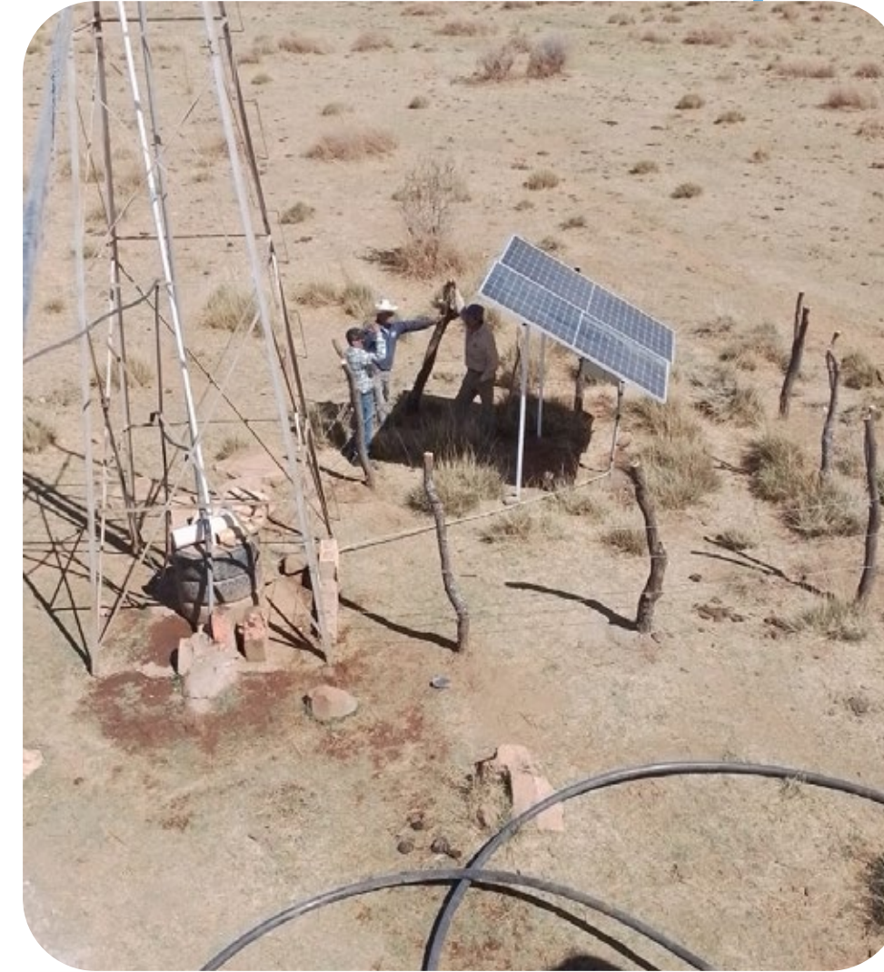
Solar powered pump at San Sebastian
