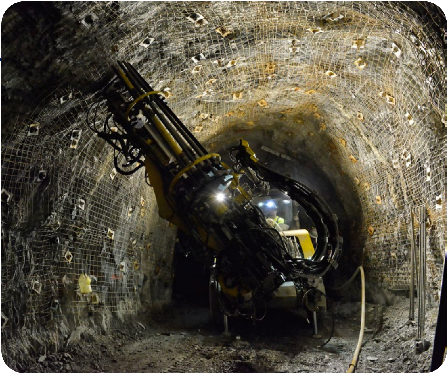
Underground rock bolter, Lucky Friday mine
